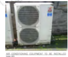
AIR CONDITIONING EQUIPMENT TO BE INSTALLED HERE
